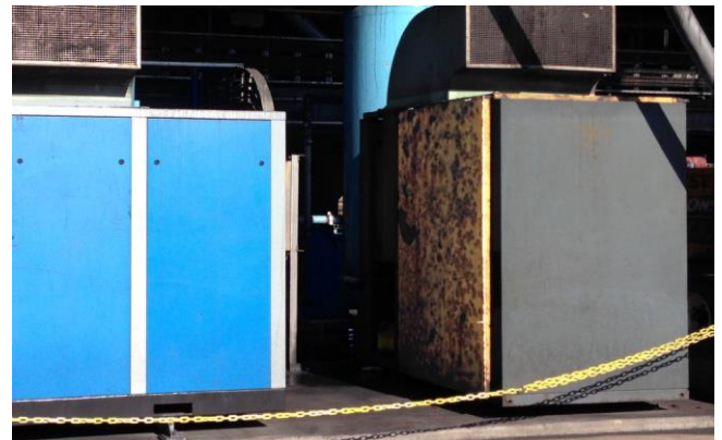
SCR Compressor stainless steel vs rusted Kaeser Compressor
