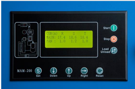
Image 2: Controller shows running amps.
