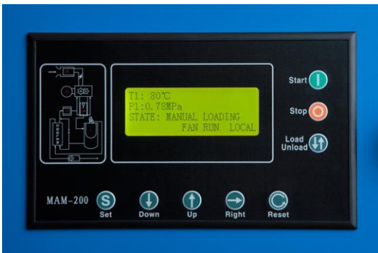
Image 1: Controller shows on load running
